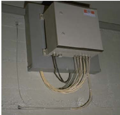
Figure 5: Local connection box
