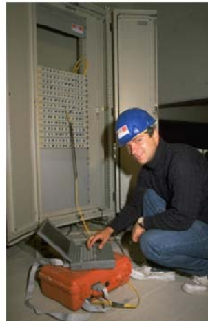
Figure 6: Central connection box
